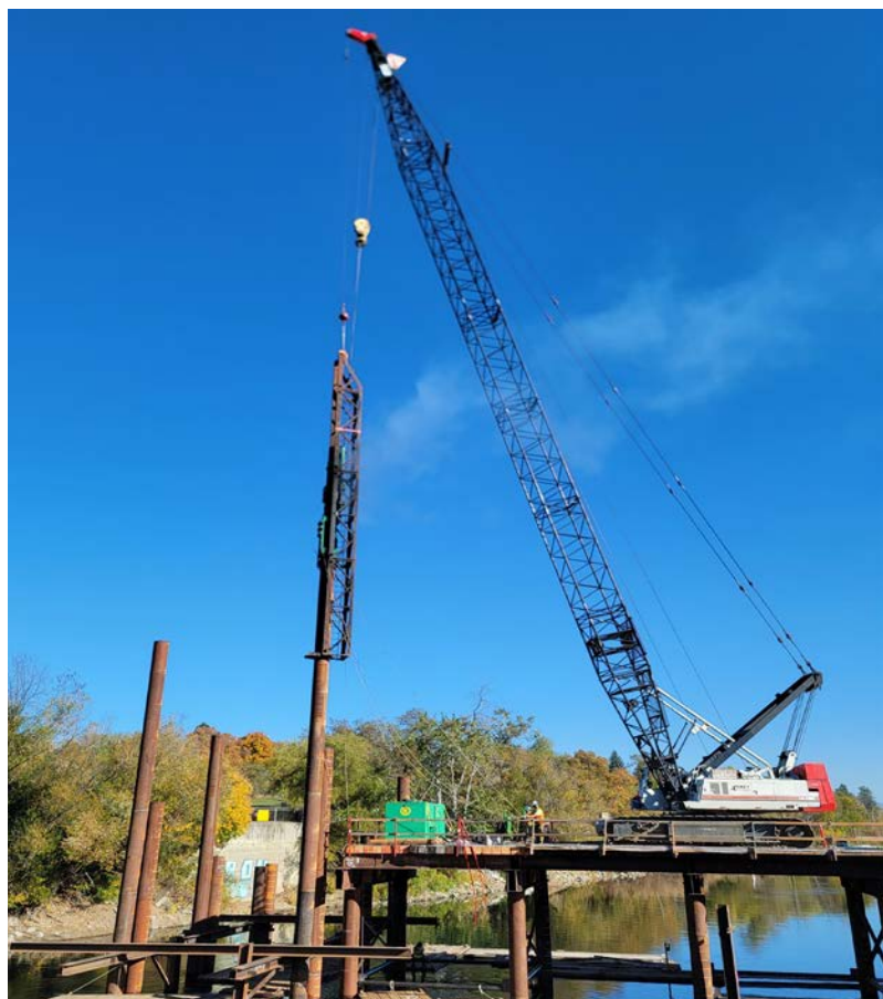
Local 302 member Mike Brotnov running a Link-Belt 238 crane driving pile for a temporary bridge over the Spokane River as part of the North Spokane Corridor project
