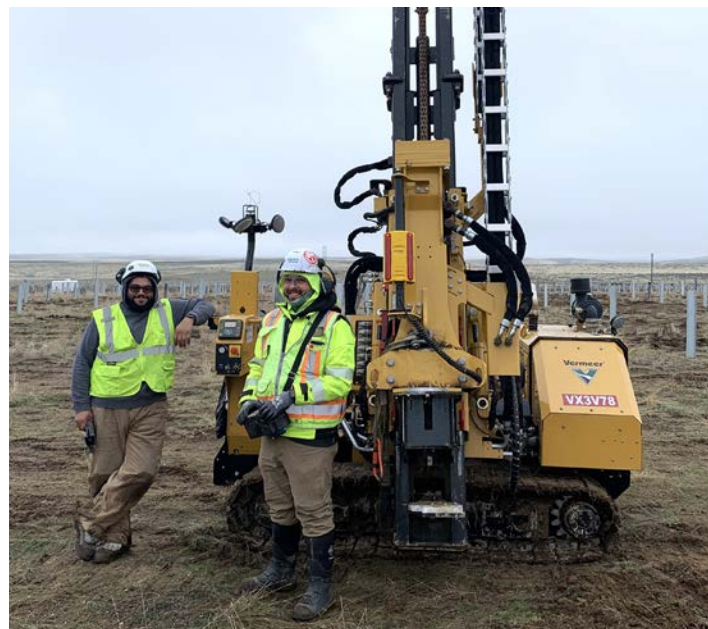
From left to right: Members Israel Escalera and John Sosa take a break from operating the Vermeer PD10 to drive substructure posts into the ground for the solar panel mounting framework at the Goose Prairie project
