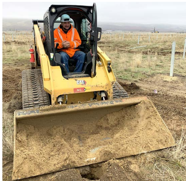
Member Kenny Melton operates a skidsteer on the fill crew who fills the pre-drilled holes with material the posts get driven into at the Goose Prairie project
