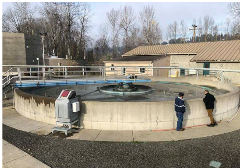
Local 302 member Andrew Silveria and IUOE District 286 District Representative Tony Frascone view a primary clarification tank in operation
